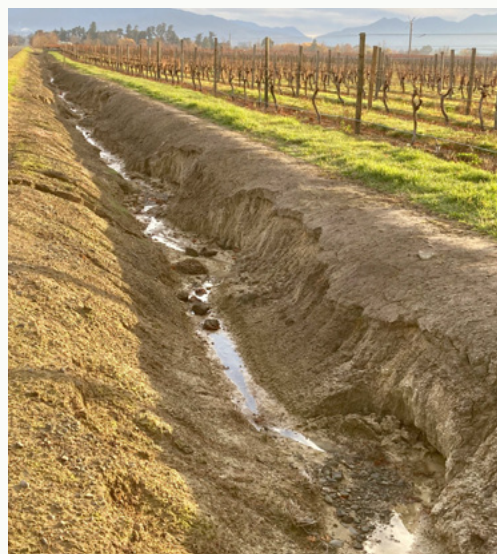
Erosion and sedimentation in a sprayed-out drain
